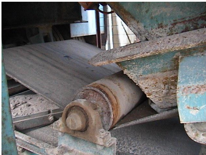
2: The conveyor belt-roller of the machine.
